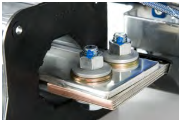
Figure 4-8. Check the bus bar connections
