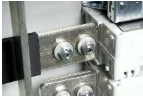
Figure 4-4. Inspection of the bus bar connection
