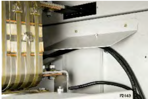
Figure 4-3. Air deflector check
