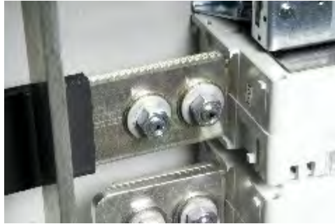
Figure 4-1. Bus bar terminal and connection
